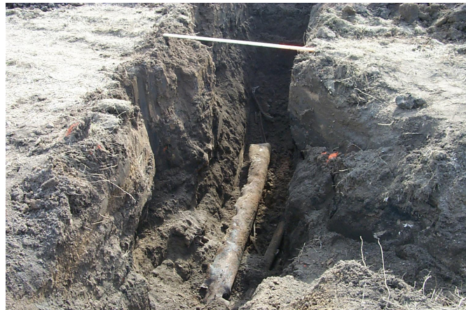
Figure 7. Anomaly two at point (65, 161) was caused by a junk steel pipe. A 3-ft stick serves as a scale.
