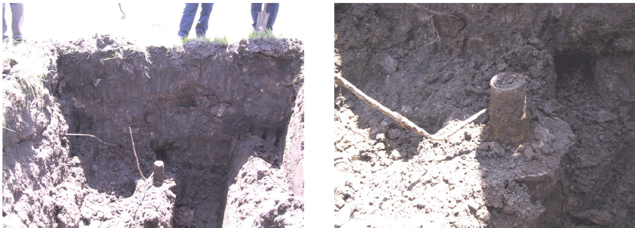
Figure 6. The abandoned brine well was unearthed. Observers' legs serve as a scale (left). This well is located at point (110, 40). A close-up photo is on the right.
